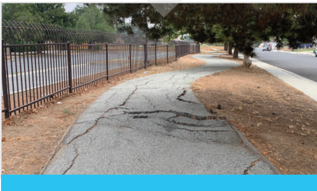
Lifted Asphalt in Bike Path Due to Invasive Tree Roots
