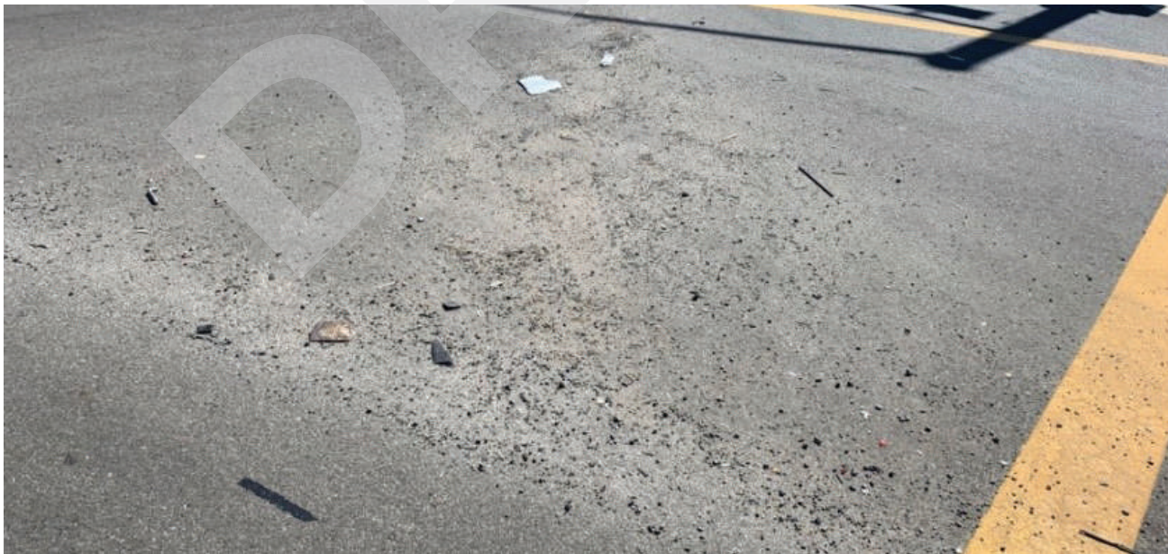
Triangular Shaped Debris Area with an Intersection
