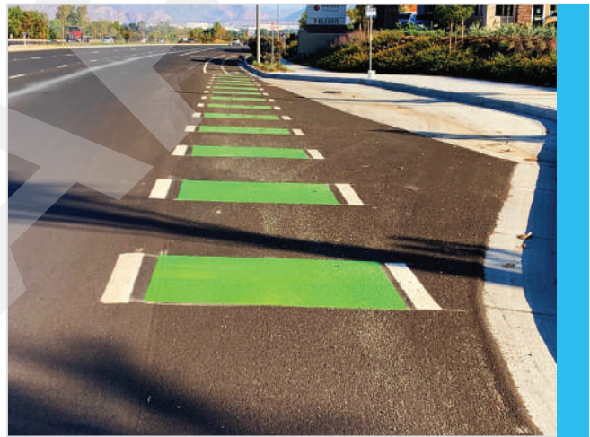
Conflict Markings at Bus Turnout
