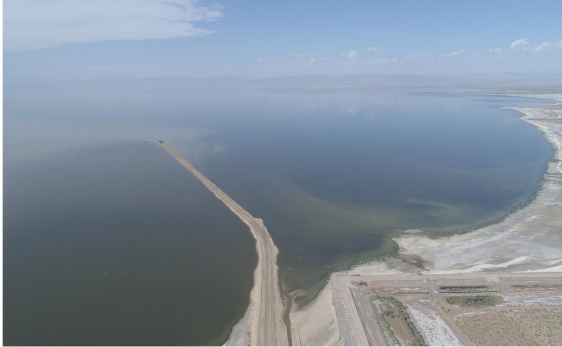
Completed causeway to the saline pump station, looking north toward the Salton Sea from the New River.
