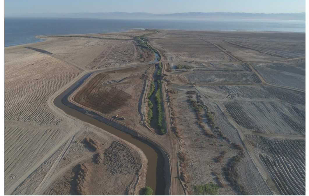
New River diversion to allow construction of the of intake structure for the SCH.
