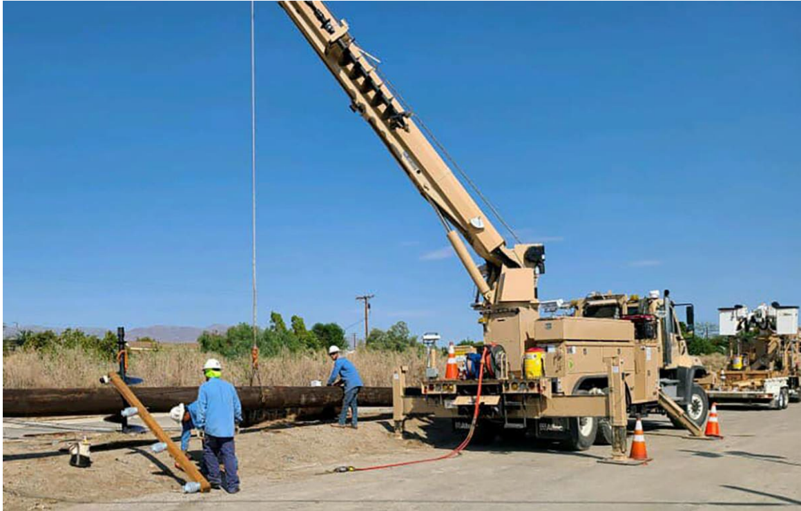
IID's energy crews work to set a new power pole in the Coachella Valley.
